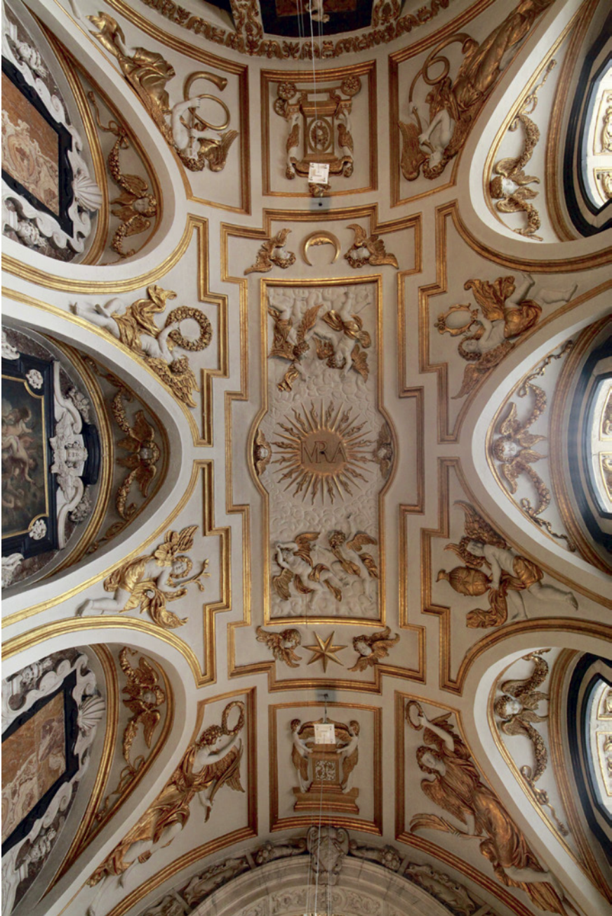
FIGURE 8.15 Ceiling with gilt stucco decoration, attributed to Andries de Nole, c. 1631, chapel of the Virgin, Carolus Borromeuskerk (former Jesuit church), Antwerp PHOTO: AUTHOR
